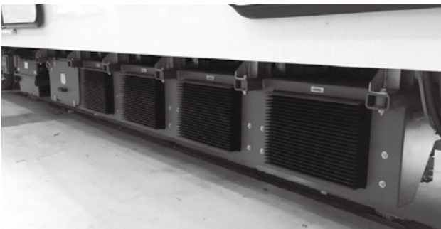
Fig. 7—Traction Converter Layout. The aluminum inverter heat sinks in the train underfloor are cooled by air flow due to train movement.
