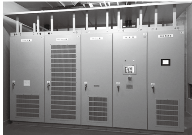
Fig. 6—Chopper Panel (with Auxiliary Power Supply Panel at Far Right). The photo shows the chopper panel and the auxiliary power supply panel, which provides the self-sufficient power supply function for auxiliary devices.
