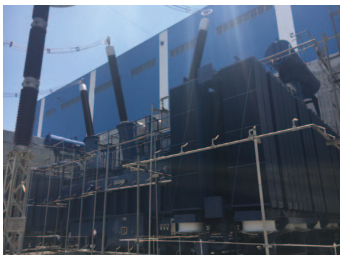
3 Transformer in operation
