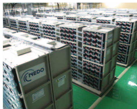
10 LL-G lead-acid batteries installed on Izu Oshima
