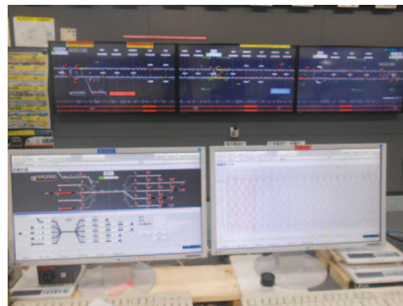
7 Rail service display panels used by Okinawa Urban Monorail's traffic management system
