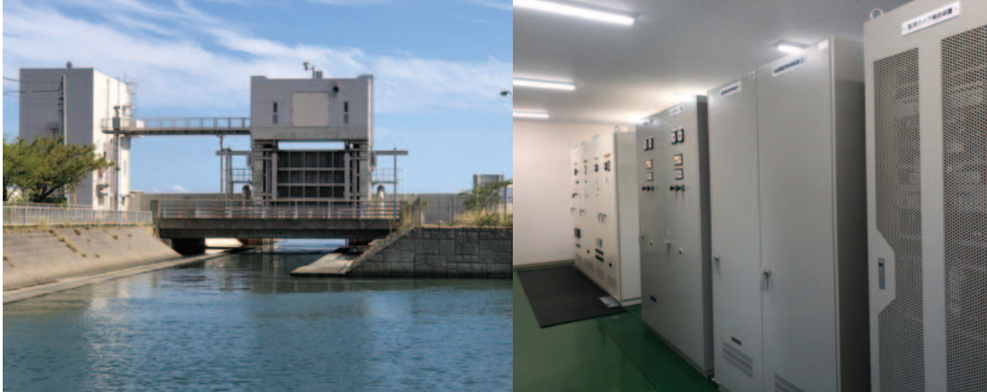
1 Panoramic view of Segami River's tsunami gate (left) and the remote monitoring system at Hitachi District Office (right)
