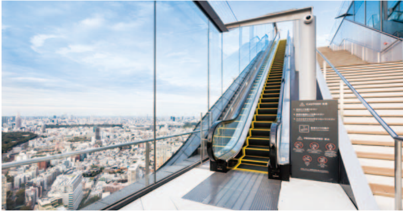
7 Outdoor escalator installed in the rooftop observation space of Shibuya Scramble Square
