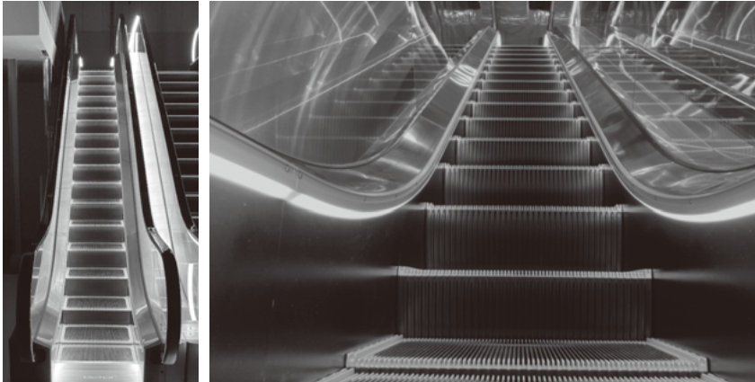
Figure 4 — Skirt Mold Lighting
