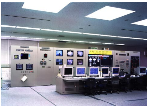
Fig. 5—View of Main Operator Control Panel and Expanded-Display Devices in Central Control Room.
