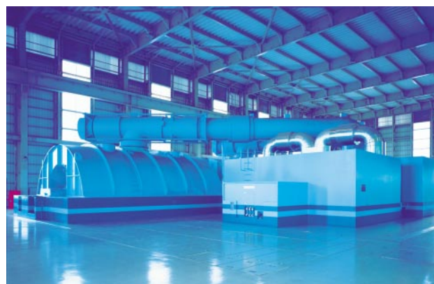
Fig. 4—View of Steam Turbine-generator Facility. Completed steam turbine-generator applying the latest technology is shown.
