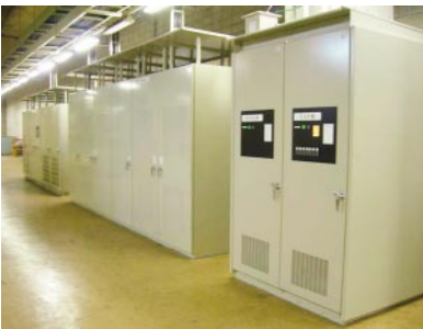
Fig. 5—Regenerative Energy Absorbing Equipment Using Batteries. Installed in substations along the wayside, the regenerative energy absorbing equipment using batteries stabilizes supply voltages and improve regenerative efficiencies.
