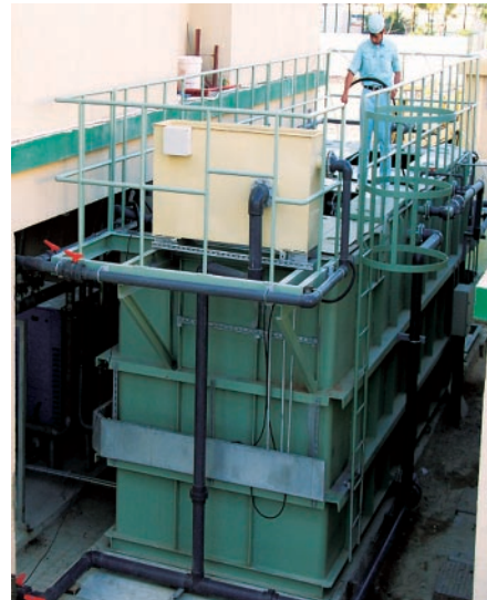
Fig. 9—MBR Facility for Construction-worker Camps. The appearance of an MBR facility installed at a construction-worker camp in Dubai City in 2007. The facility has a treatment capacity of 250 m 3 /d in processing human wastewater for about 1,500 people.
