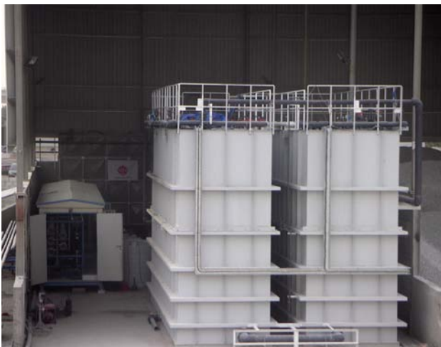
Fig.7—First Stage Plant of Water Recycling Project.
