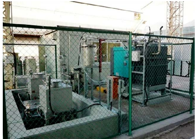
Fig. 5—40-kW Class Cycling Renewable Energy Demonstration Plant.
