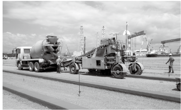
Fig. 8—Use of Slipforming to Lay Foundations. The photograph shows the concrete array foundation being laid by the Huron concrete slipform paver, which pours and forms the foundation as it moves along. The Huron machine is on the right and the concrete mixer on the left supplies it with concrete.
