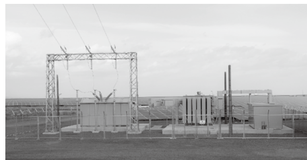
Fig. 3—Extra-high-tension Substation (Grid Connection Substation). The extra-high-tension transformer is located at the center of the extra-high-tension substation. The lines to the transmission pylon run via the gantry.
