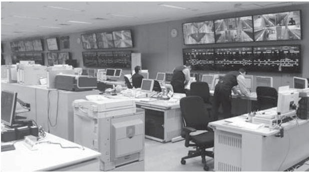
Fig. 2—Control Room at Integrated Control Center. Monitoring and automatic control of all trains on the four lines are performed by using the traffic display panels for each line, which are mounted side-by-side in the control room and at the supervisory control desks.
