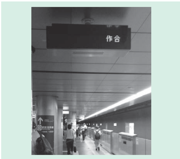
Fig. 7—Notification Display (Horizontal). These are installed between the middle and far end of the platform to provide operating instructions to the conductor and station staff.
