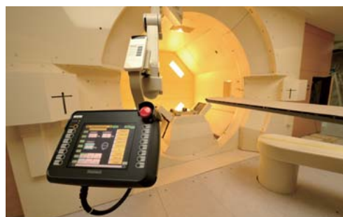
Treatment room with molecular tracking proton beam therapy system (prior to completion of installation). The system is designed to be easy for hospital staff to use.
