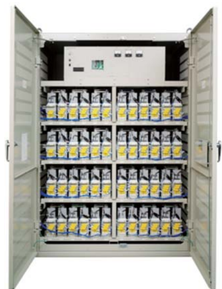
2 Lithium-ion storage battery system (maximum continuous electrical discharge 500 A)
